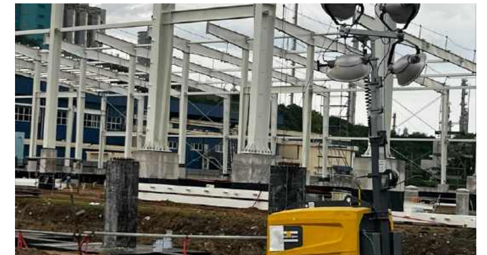
Electrical Supply for GAD Builders
