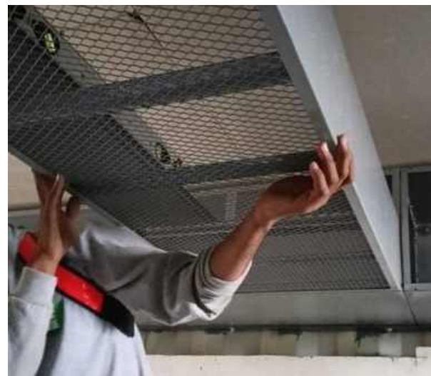
Cable Tray Supply
